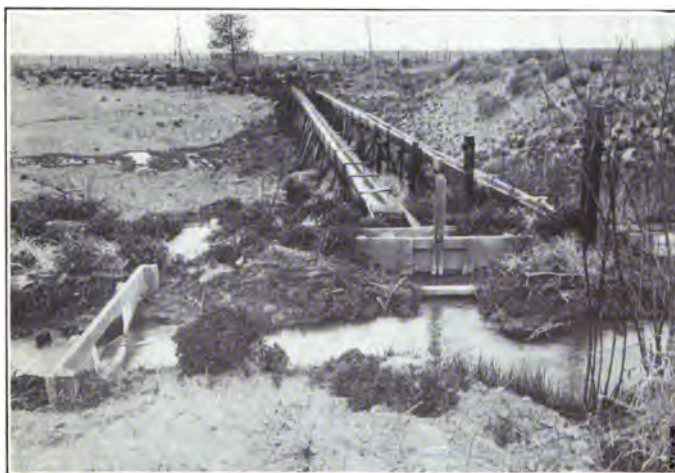
FARMER'S WOODEN HEADGATE. Small flume and measuring weir at left.
